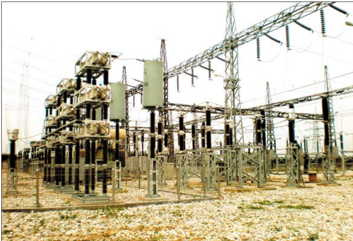
《Capacitor Bank 150kV 25Mvar – GI Duri substation in Indonesia》
